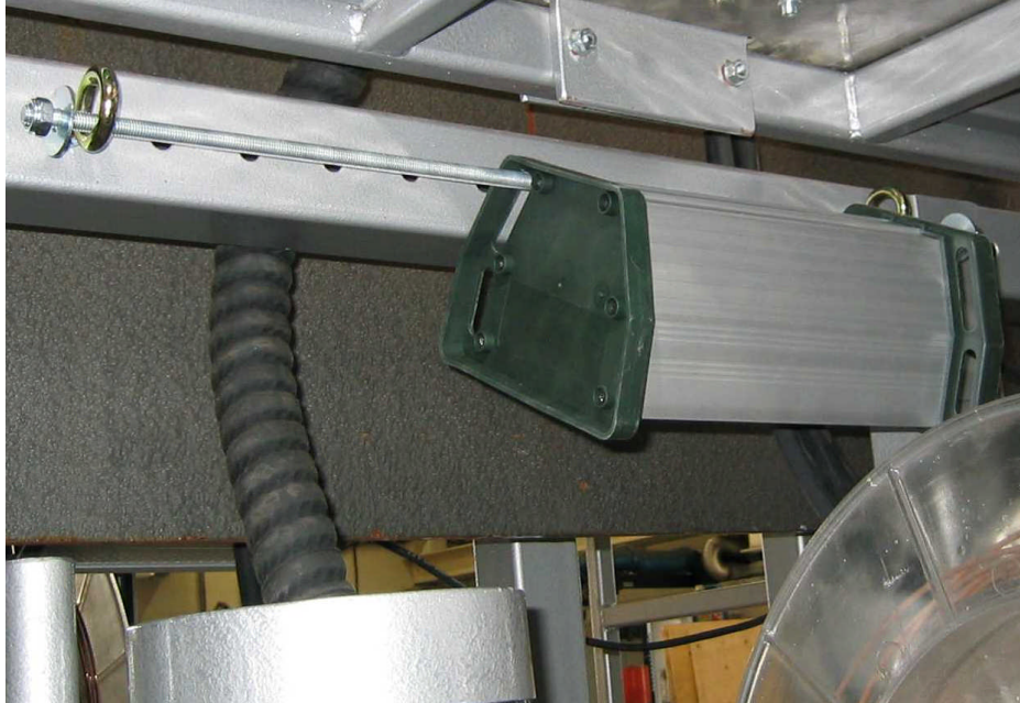
Fig. Lamp installed in the cabin.
